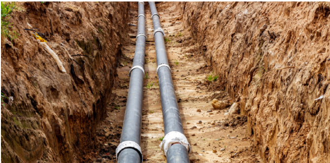
Lead Water Line Replacement | Project funded by 3rd Ward residents through PB
